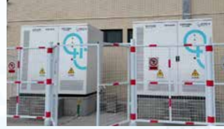
◆ Delong Manufacturing Tech Park Project Location: Guangdong Province, China Scale: 480kW/930kWh
