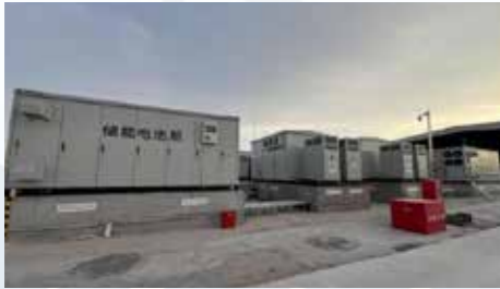
◆ Lianyungang Donghai 50MW/100MWh Energy Storage Power Station Project Location: Jiangsu Province, China Scale: 50MW/100MWh
