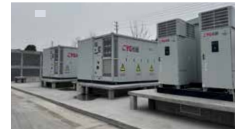
◆ Jiangsu Shenyuan Group 10MW/20MWh Energy Storage Station Location : Taizhou, Jiangsu Scale: 10MW/20MWh
