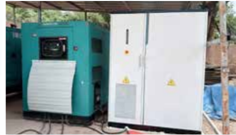
◆ 125kW/225kWh Energy Storage Project in Guinea Location: Guinea Scale: 125kW/225kWh
