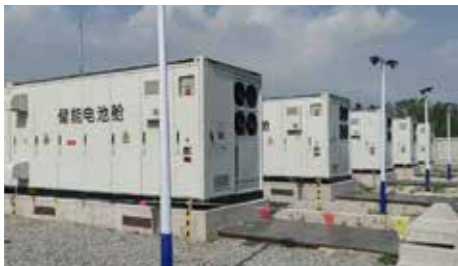
◆ Ganyu District 50MW/100MWh Independent New Energy Storage Power Station Location: Jiangsu Province, China Scale:50MW/100MWh
