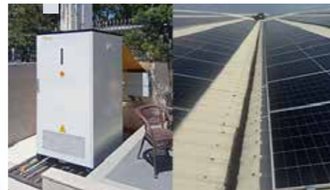
◆ 267.84kW Photovoltaic + 250kW/400kWh Energy Storage Project in the Philippines Location: Philippines Scale: 250kW/400kWh
