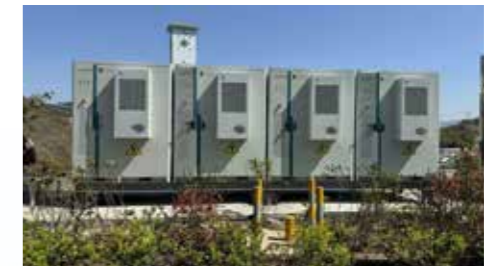
◆ Hangzhou Fuyang Huilong Environmental Technology Co., Ltd. Energy Storage Project Location: Hangzhou, Zhejiang Province Scale: 400kW/800kWh
