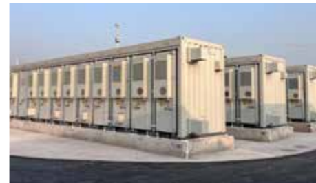
◆ Jurong Huayang 100MW/200MWh Shared Energy Storage Power Station Location: Jiangsu, China Scale: 100MW/200MWh
