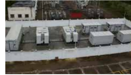
◆ Ziyang Virtual Power Plant Green Demonstration Application Project Location: Ziyang, Sichuan Province Scale: 25MW/50MWh
