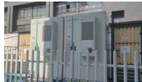
◆ Zhejiang Yiwu Zhuopin Energy Storage System Project Location: Yiwu City, Zhejiang Province Scale: 200kW/400kWh
