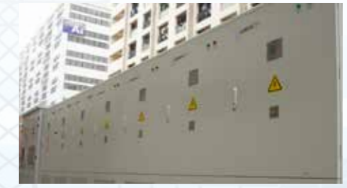
◆ Dongguan Zhongchuang Zhibang Industrial Park User-Side Energy Storage Power Station Project Location: Guangdong Province, China Scale: 1.118MW 2.236MWh
