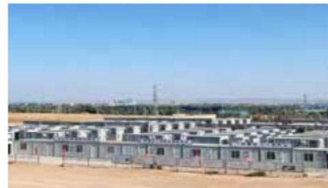
◆ Shangchu Energy Independent shared Energy Storage PowerStation Location: Ningxia, China Scale:100MW/200MWh
