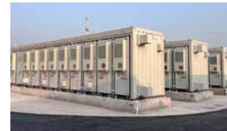
📍 Jurong Huayang 100MW/200MWh Shared Energy Storage Power Station Location: Jiangsu, China Scale: 100MW/200MWh
