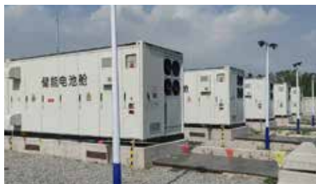
📍 Ganyu District 50MW/100MWh Independent New Energy Storage Power Station Location: Jiangsu Province, China Scale:50MW/100MWh
