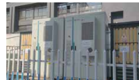
📍 Zhejiang Yiwu Zhuopin Energy Storage System Project Location: Yiwu City, Zhejiang Province Scale: 200kW/400kWh
