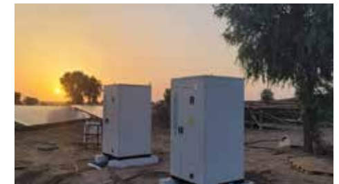
📍 India 0.5~3MWh C&I BESS Location: India Scale: 0.5~3MWh
