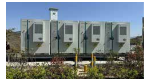
📍 Hangzhou Fuyang Huilong Environmental Technology Co., Ltd. Energy Storage Project Location: Hangzhou, Zhejiang Province Scale: 400kW/800kWh
