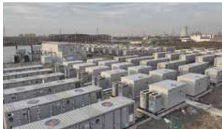
📍 Lianyungang Energy Group Independent and Shared New Energy Storage Project Location: Jiangsu Province, China Scale: 150MW/300MWh
