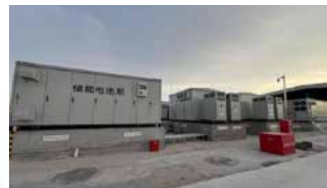
📍 Lianyungang Donghai 50MW/100MWh Energy Storage Power Station Project Location: Jiangsu Province, China Scale: 50MW/100MWh
