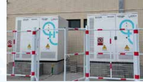
📍 Delong Manufacturing Tech Park Project Location: Guangdong Province, China Scale: 480kW/930kW
