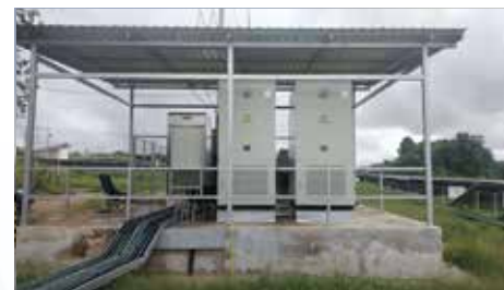
📍 Laos 1.25MW/2.61MWh Solar-plus-Storage Project Location: Laos Scale: 1.25 MW/2.61 MWh
