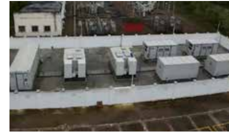
📍 Ziyang Virtual Power Plant Green Demonstration Application Project Location: Ziyang, Sichuan Province, China Scale: 25MW/50MWh
