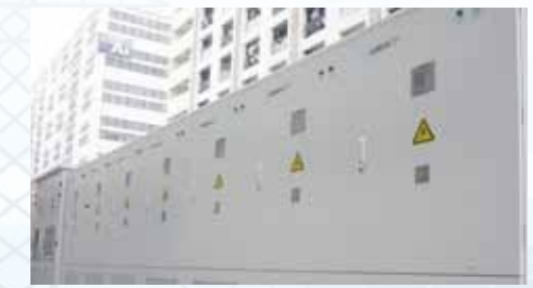
📍 Dongguan Zhongchuang Zhibang Industrial Park User-Side Energy Storage Power Station Project Location: Guangdong Province, China Scale: 1.118MW 2.236MWh
