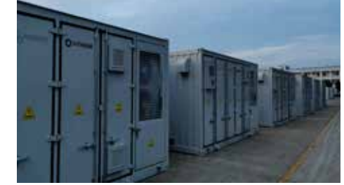
📍 China Electric Power Construction Group Jilin Institute invests in the (Ningxia) Chiyang Yanchi County 100MW/200MWh Energy Storage Power Station Location: Ningxia, China Scale: 100MW/200MWh
